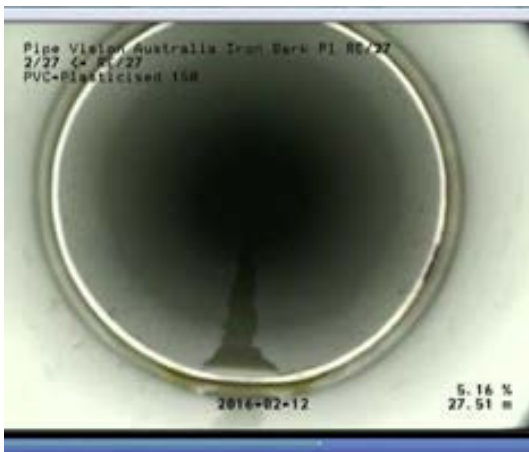
FIG A5.8: Example of excessive width at a joint - not acceptable
