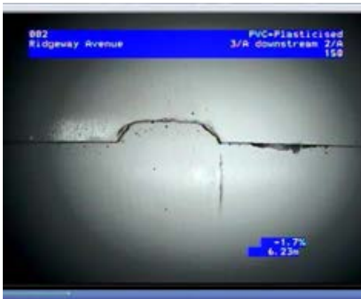
FIG A5.1: Example of a defect at a joint – not acceptable
