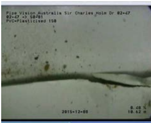
FIG A5.3: Example of a defect at a joint – not acceptable
