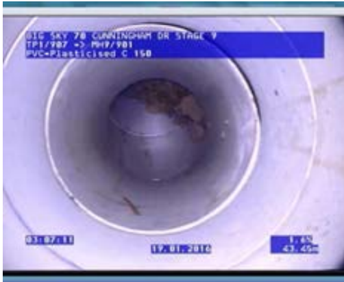
FIG A8.7: Example of a deposits in a junction – not acceptable.
