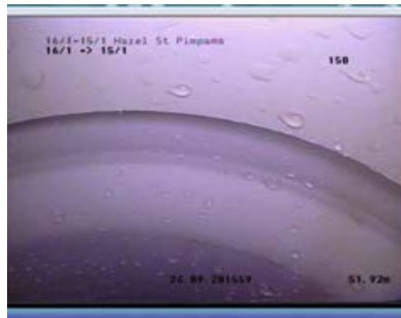
FIG A5.9: Example of excessive width at a joint - not acceptable
