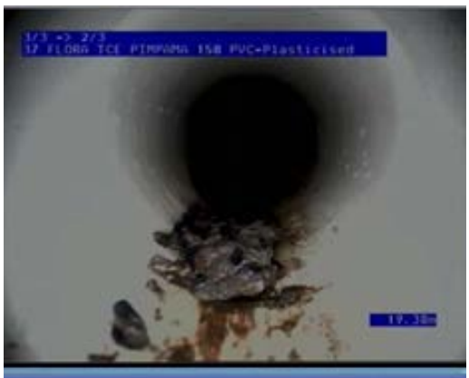
FIG A8.5: Example of a major deposits at the invert – not acceptable
