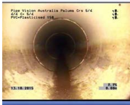
FIG A8.2: Example of a not clean pipe – not acceptable
