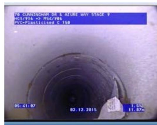
FIG A6.4: Example of an obstruction within a pipe – not acceptable
