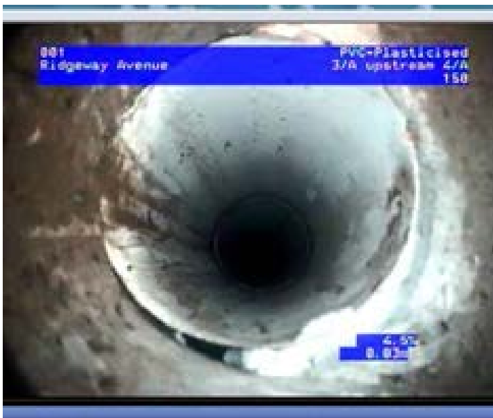
FIG A5.6: Example of a defect at the manhole/pipe interface joint – not acceptable
