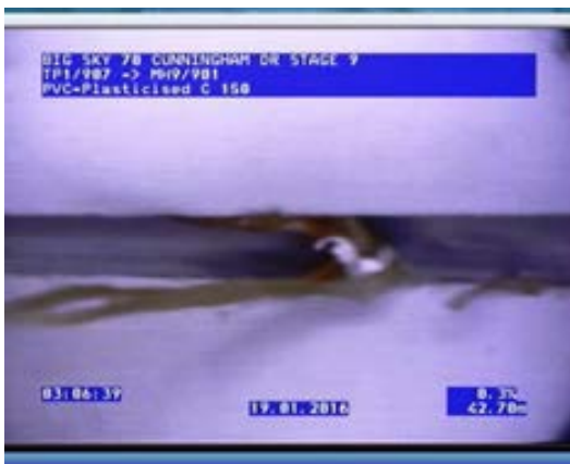
FIG A6.3: Example of an obstruction within a joint – not acceptable
