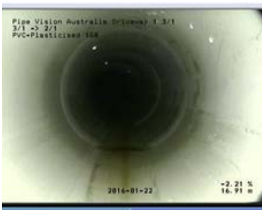
FIG A7.1: Example of minor ponding within a pipe – acceptable
