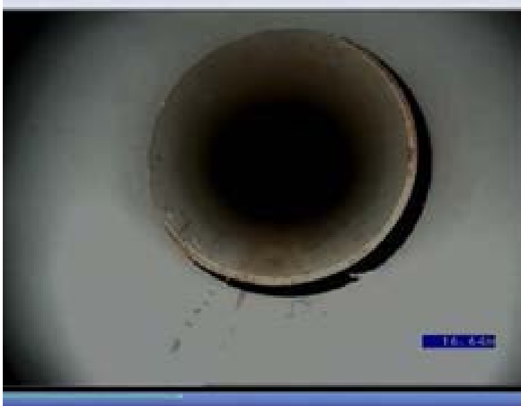
FIG A4.1: Example of collapse at a joint – not acceptable
