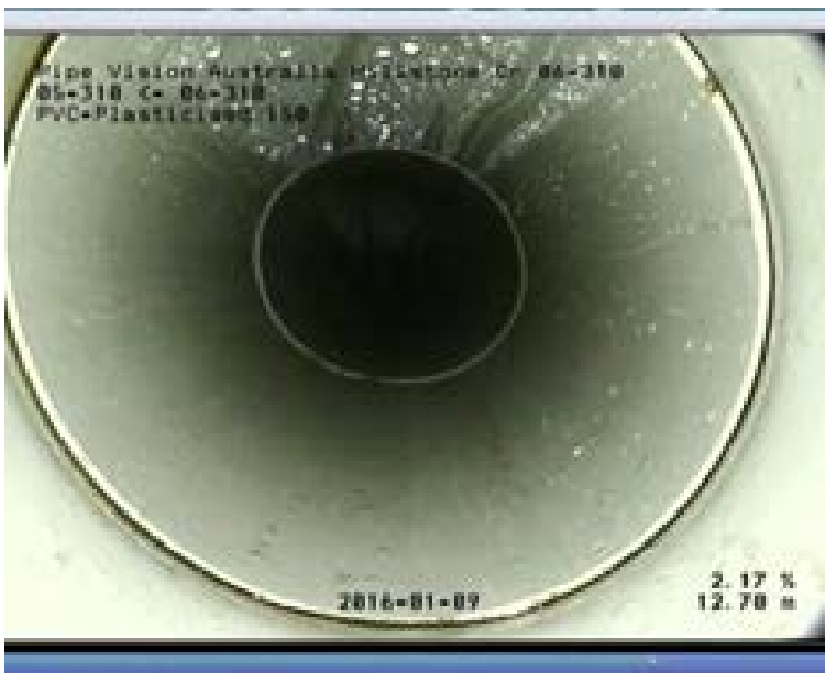
FIG A4.2: Example of deformation (ovality) – not acceptable
