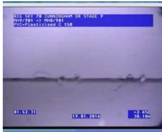
FIG A5.2: Example of defects at a joint – not acceptable
