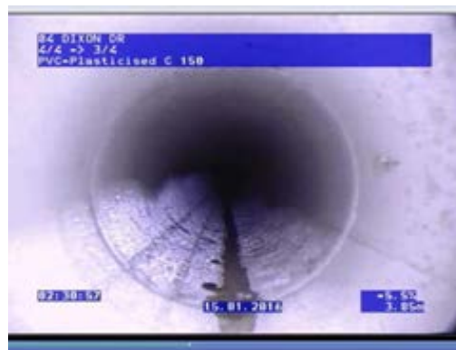
FIG A1.4: Example of poor quality footage of a joint - not acceptable
