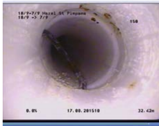
FIG A6.2: Example of an obstruction (rolled rubber) – not acceptable
