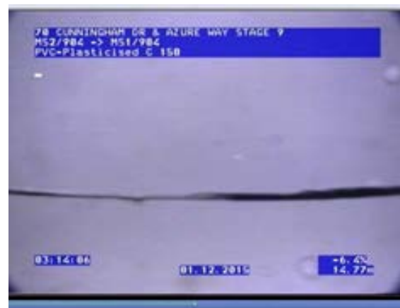
FIG A5.11: Example of no gap at a coupling - not acceptable
