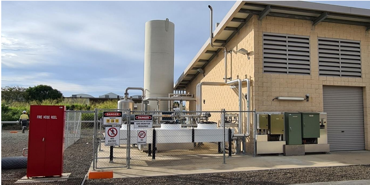
Figure 21. Fences give separation between combustible gases and ignition sources.
