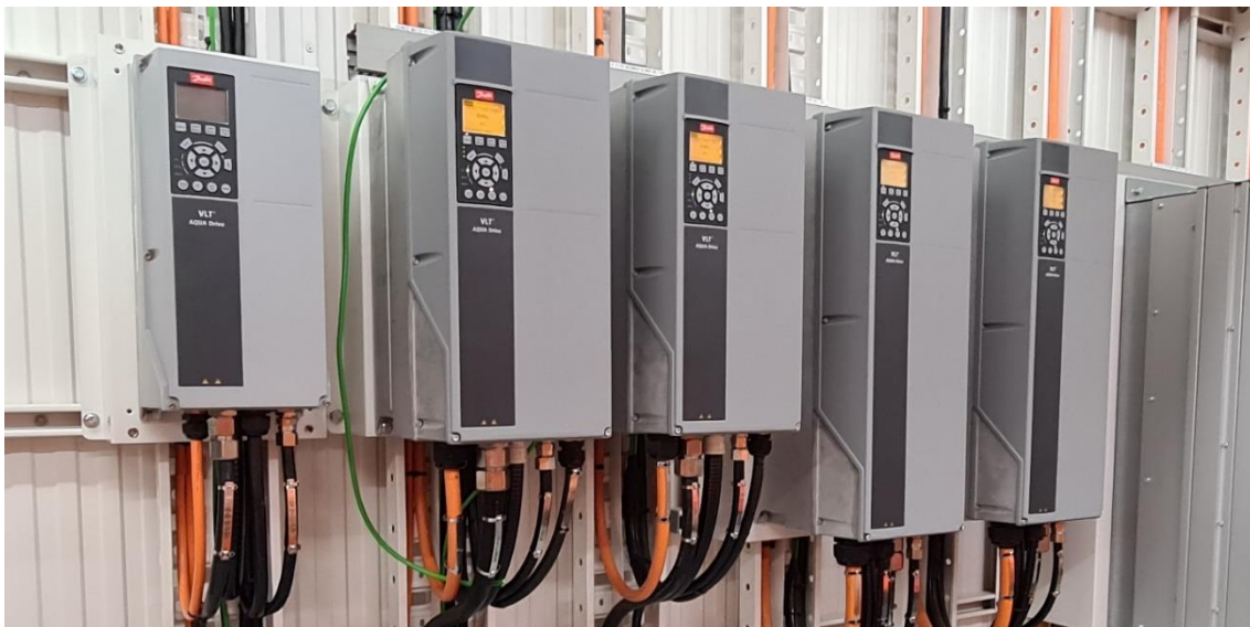
Figure 11. VSDs mounted on a wall can be lifted with a crane inside the switch room.
