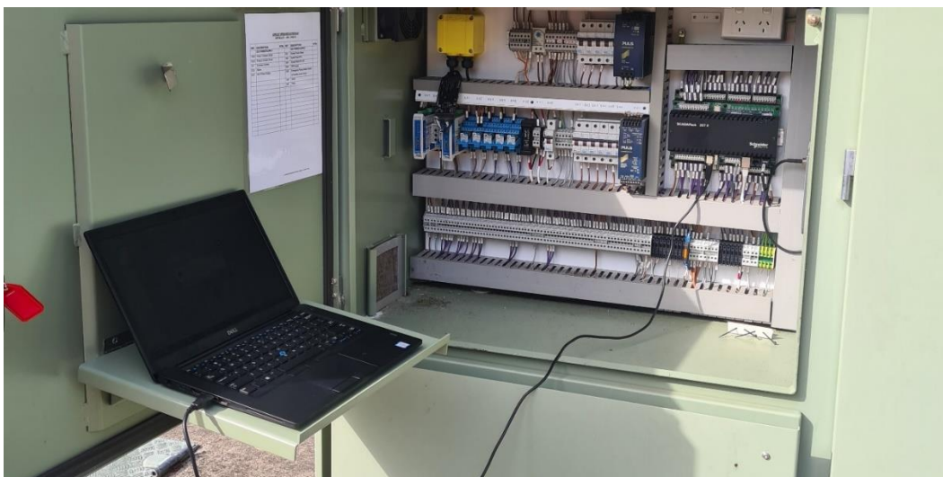
Figure 14. A laptop plugged into a control system in an ELV compartment.
