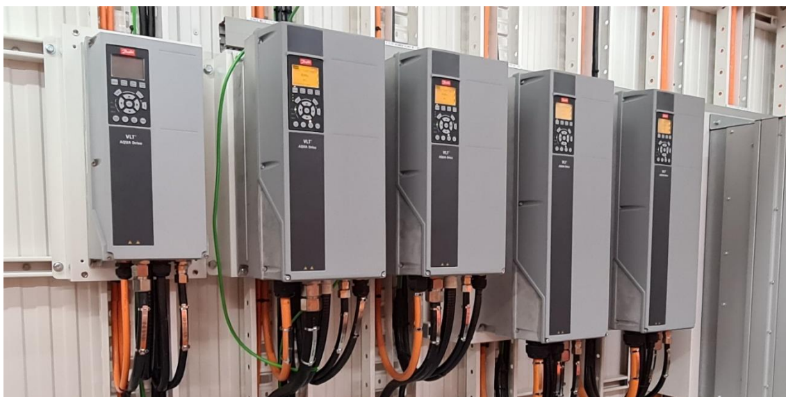
Figure 11. VSDs mounted on a wall can be lifted with a crane inside the switch room.
