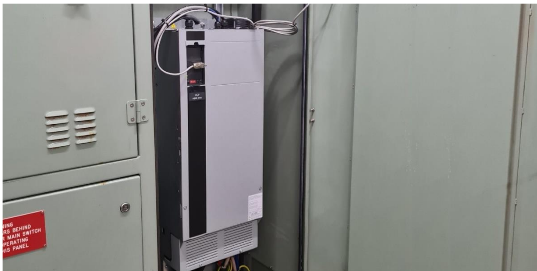
Figure 10. VSDs inside switchboards need 2 persons to manually lift and manoeuvre.
