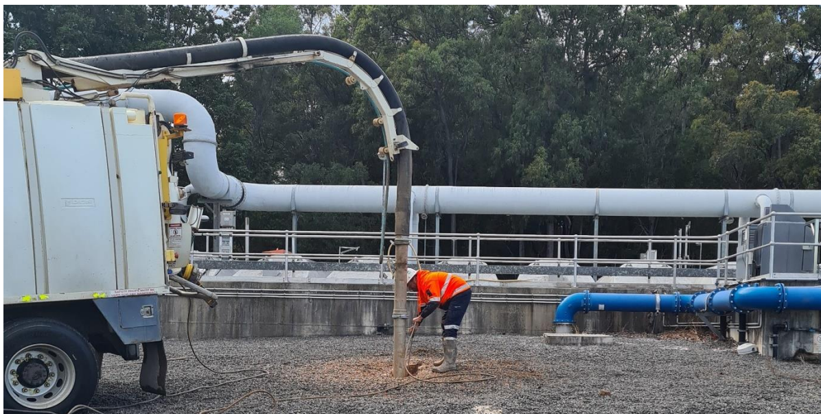
Figure 22. Pipes and conduits under gravel can be investigated when issues arise, without impacting site access.
