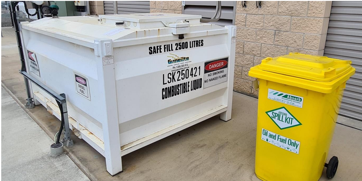
Figure 20. Combustible diesel fuel stored in an open area away from process plant.
