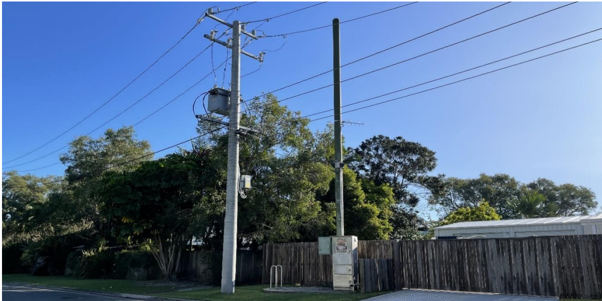
Figure 12. The pumps in this well can only be safely lifted after Energex has attended and isolated the overhead lines.
