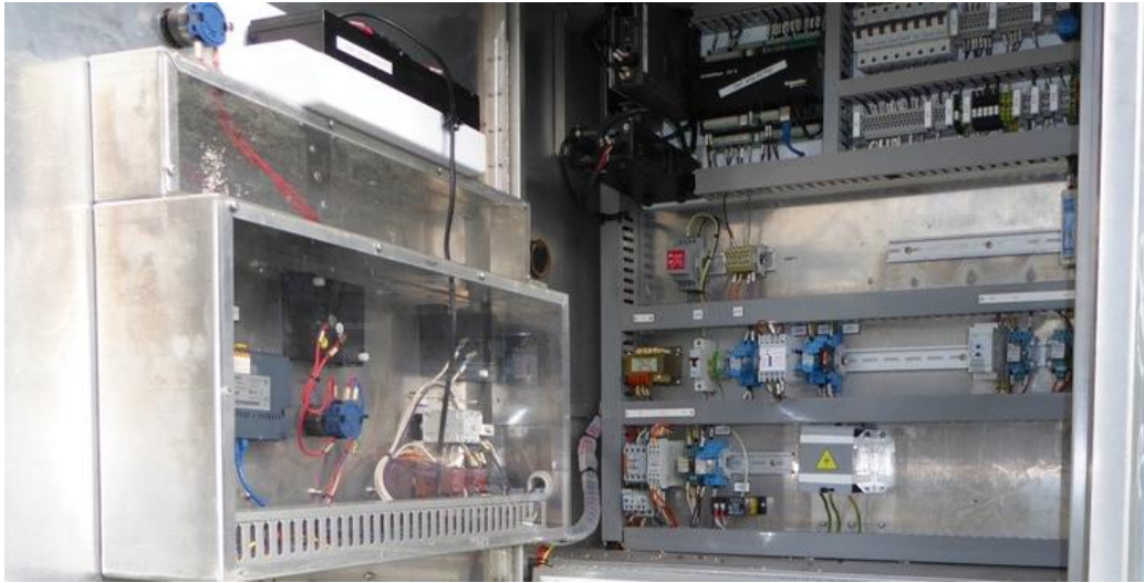
Figure 13. These ELV components (top right) should be segregated from 3 phase power.
